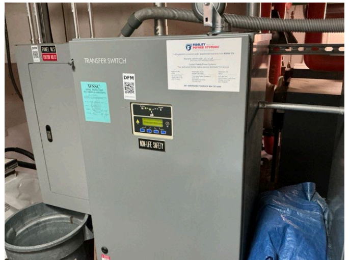
28 - AUTOMATIC TRANSFER SWITCH
