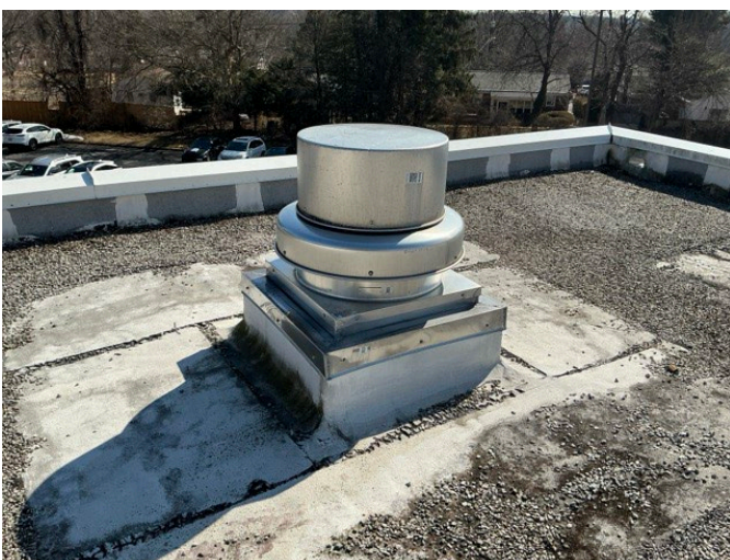
23 - TYPICAL EXHAUST FAN
