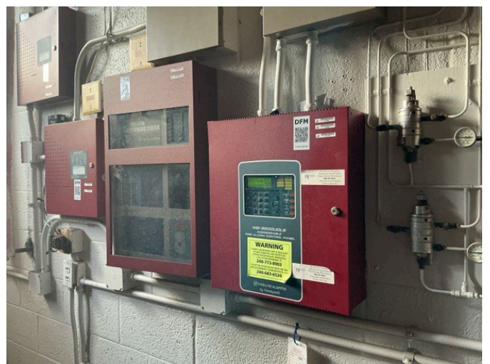
30 - FIRE ALARM PANEL
